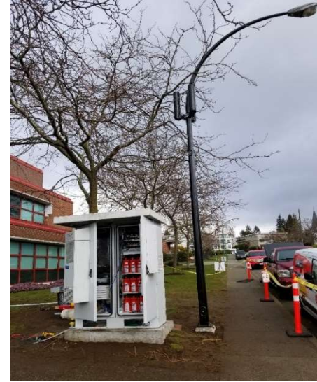
Figure 2: Antenna and Cabinet
